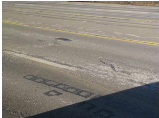
Figure 5 Typical Distress (fatigue cracking)
