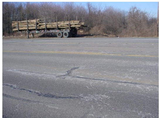
Figure 7 Typical Distress (Fatigue Cracking)
