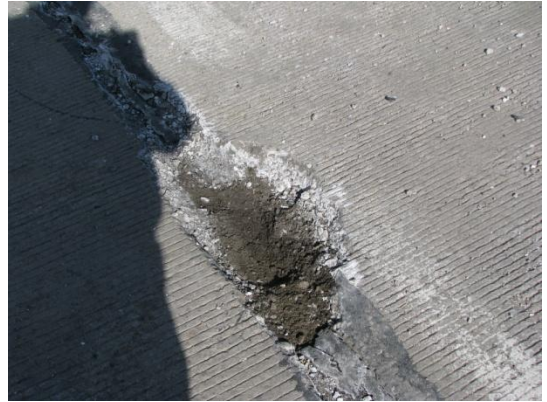
Figure 23 Typical Distress (freeze-thaw deterioration)
