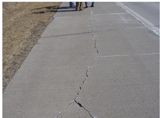
Figure 21 Subgrade Support Failure Under Shoulder
