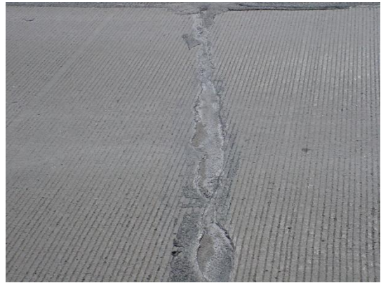
Figure 19 Typical Distress (freeze-thaw deterioration)
