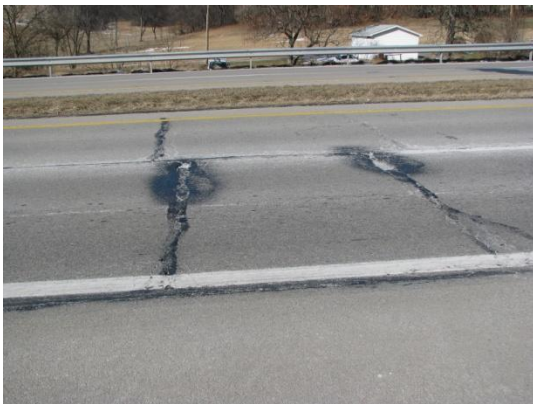
Figure 16 Typical Distress (reflective cracking) Northbound Lane
