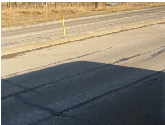
Figure 6 Fatigue Cracking with Moderate Rutting
