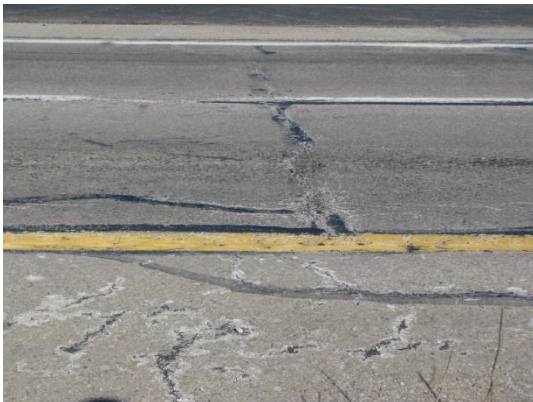
Figure 12 Typical Distress (reflective and fatigue cracking)
