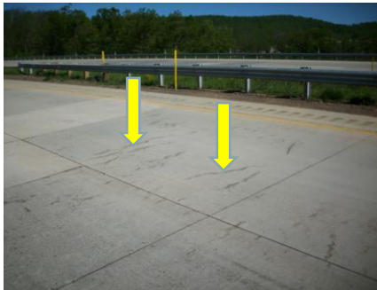
Pavement showing signs of distress
